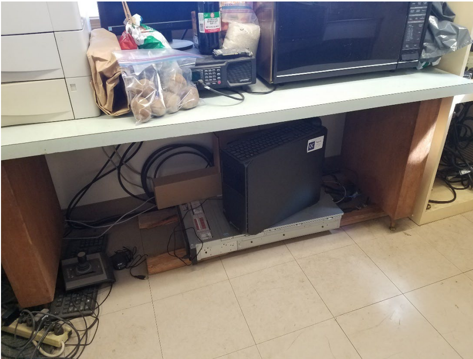
Photo 46: Existing radio equipment to be relocated.
