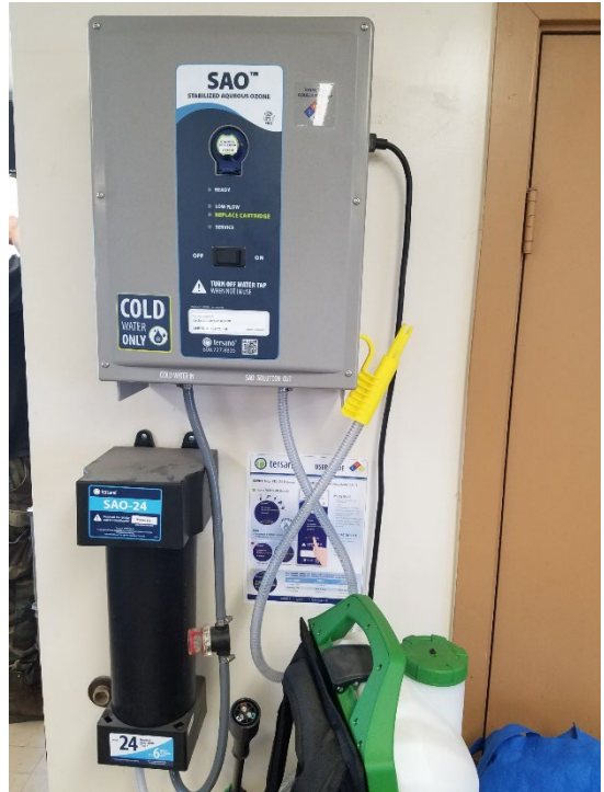
Photo 28: Existing disinfecting equipment to be relocated.
