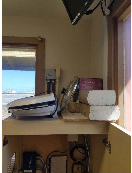
Photo 48: Existing equipment cabinet.
