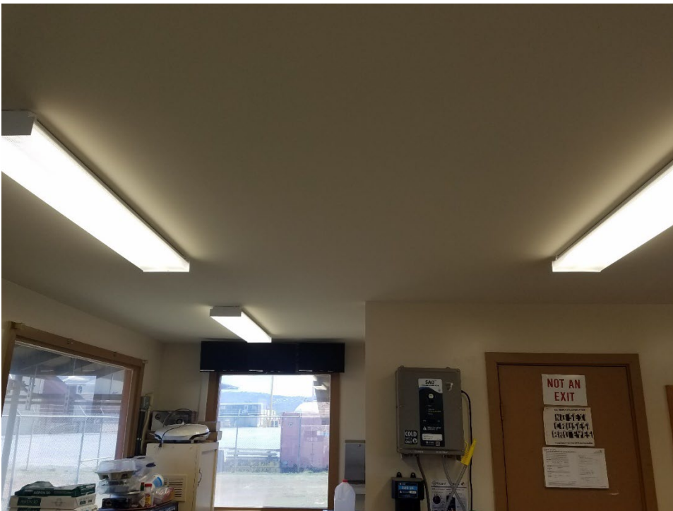
Photo 11: Office ceiling facing kitchenette.
