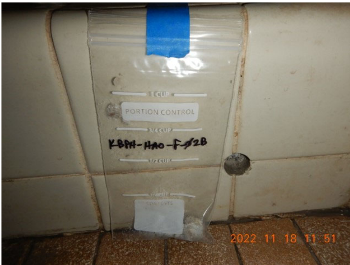
Photo 9 - KBPH-F-02B (Close-up) [AL\DSCN8374.JPG]
