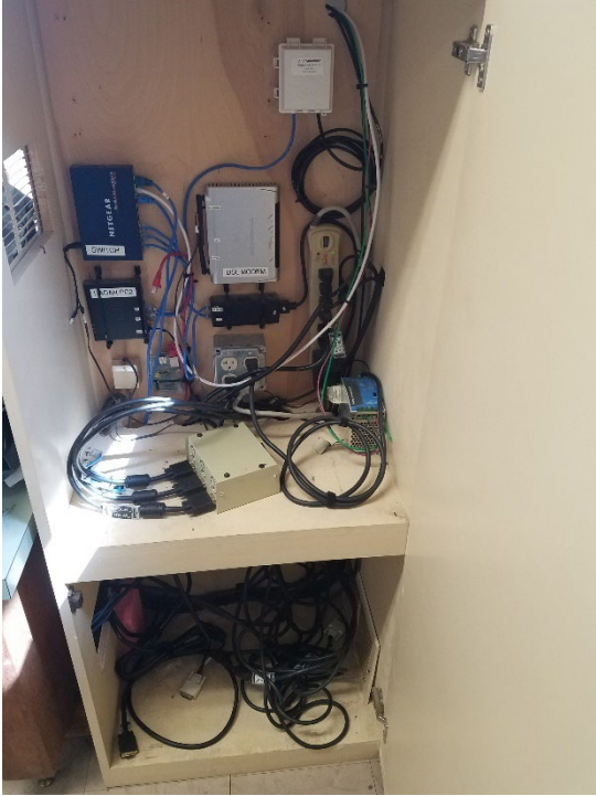
Photo 47: Existing equipment cabinet.
