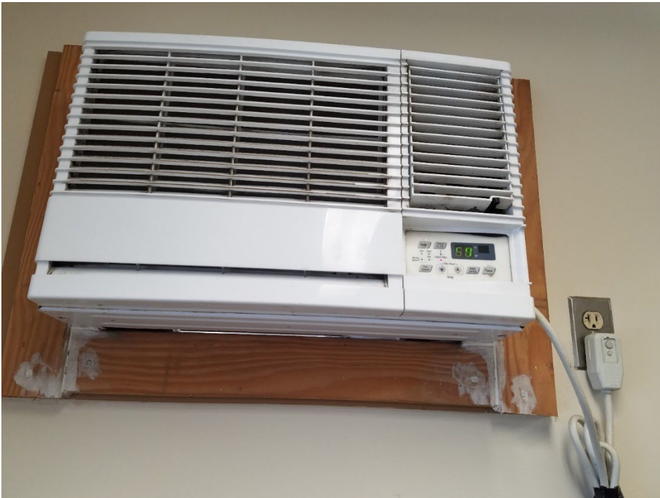
Photo 26: 1 of 2 existing through wall window air conditioners to be removed.
